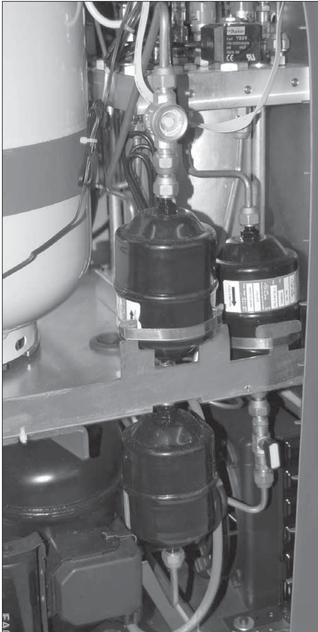
R/R/R machine internal plumbing must be periodically checked to make sure no leaks are present.
