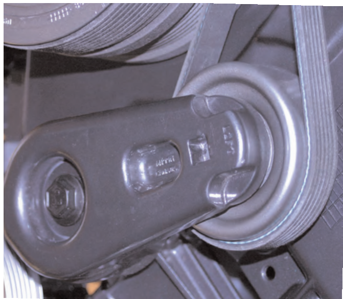
If the belt tensioner is worn, the pump will not work properly.
