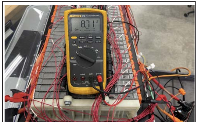
Voltage Measurement on One Module
