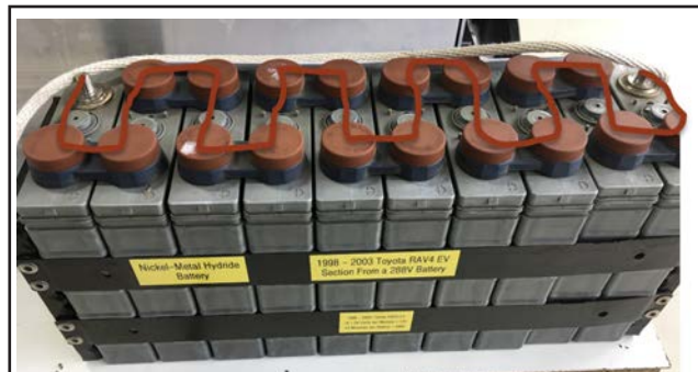
Toyota RAV 4 HV Battery Modules in Series
