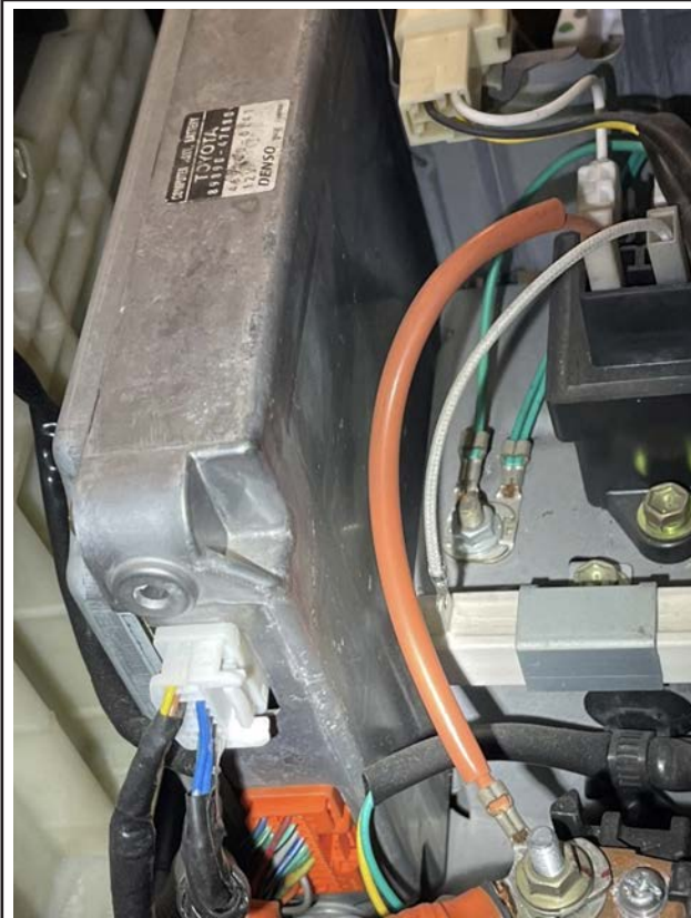
Battery Controller (Smart Unit) Gen 3 Prius
