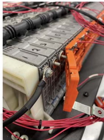
Module Test Connection Locations
