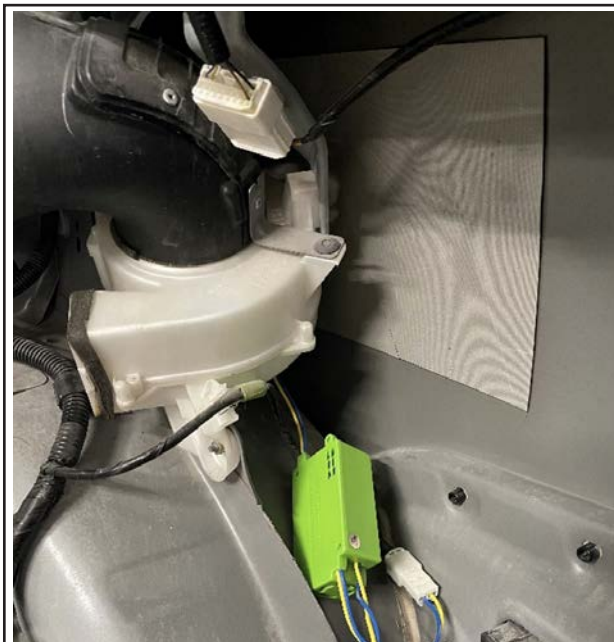
Harness Connection at Fan
